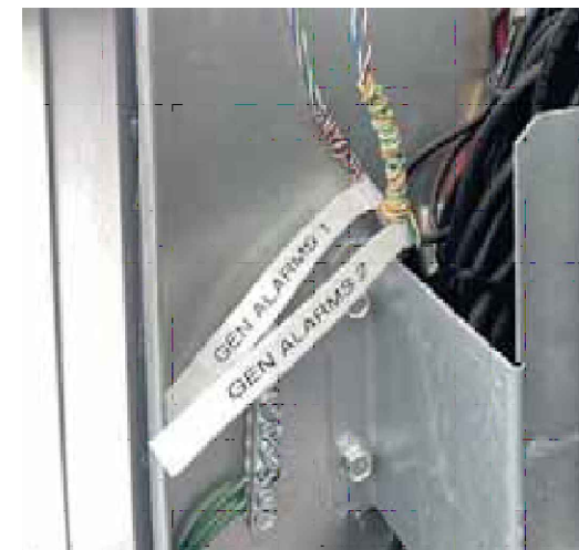
LABELS AT GENERATOR
